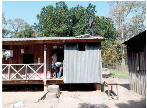
dhurba post solar installation
